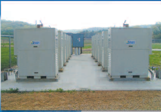
The Sauk County Landfill, located in Madison, Wisconsin, is the largest landfill microturbine installation east of the Rockies.
